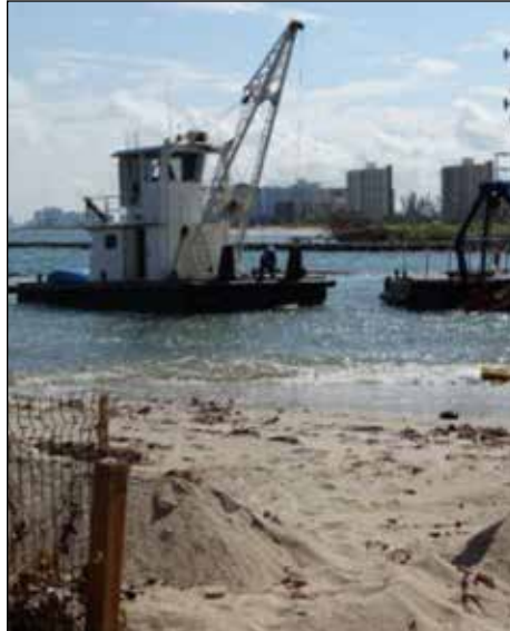
A small dredge pumps sand from a channel onto a Fort Lauderdale beach.
